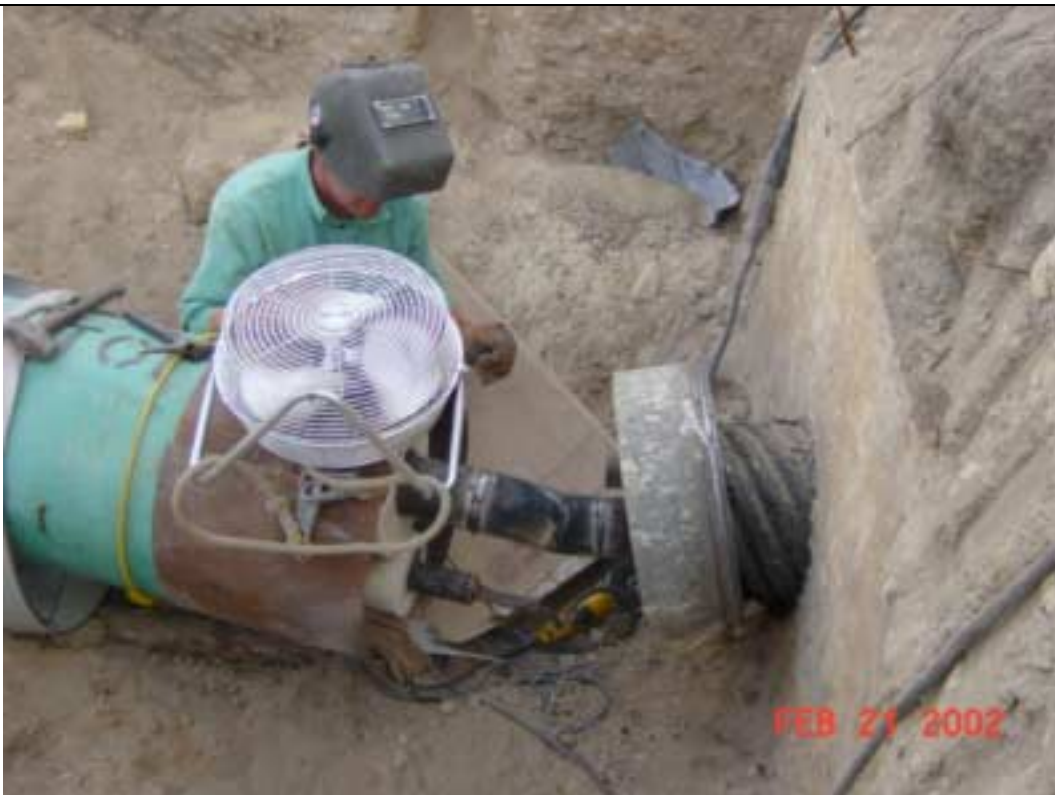
Steam bypass tie-in
