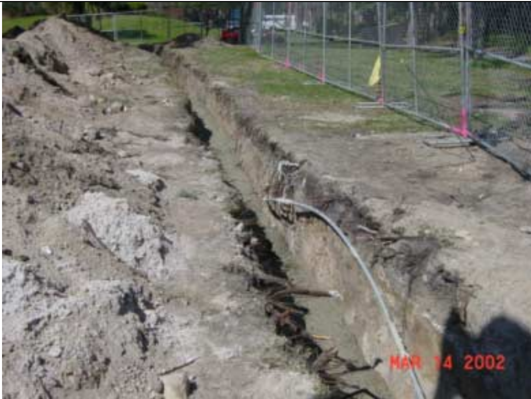
Duct bank North of Inner
