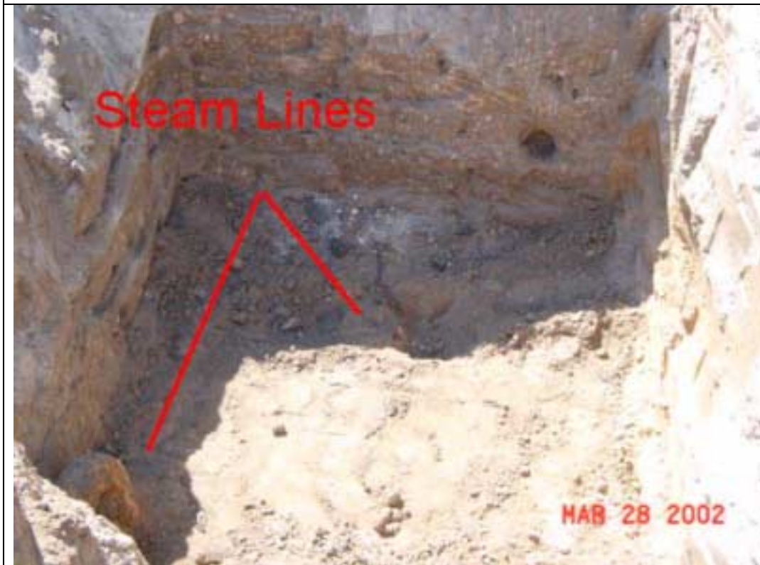
Steam Line Conflict.JPG
