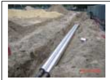
Chilled Water Piping with Field-Applied Foam Glass Insulation with Pittwrap
