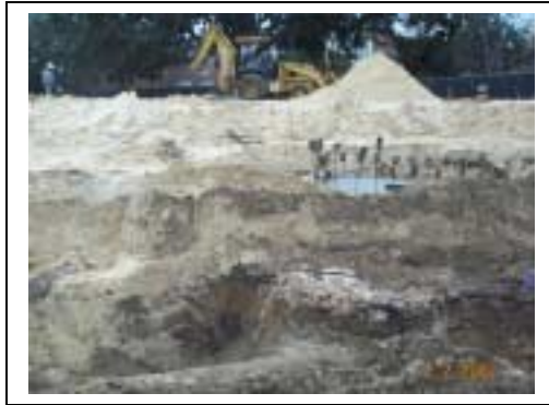
Asbestos-Coating found at Existing Steam Pipe
