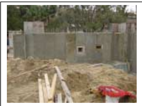
Mechanical Room Wall with Sleeves
