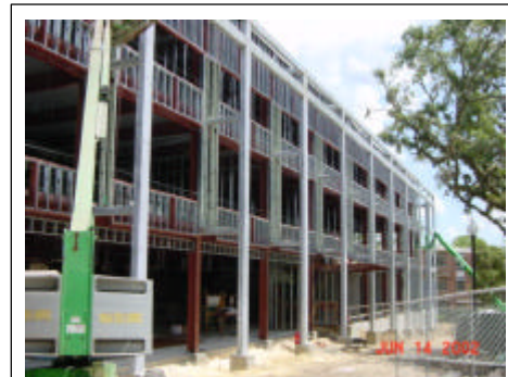
Exterior metal stud framing: substrate for the metal wall panel and glass building skin.
