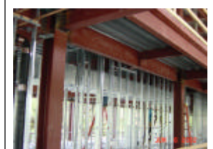
Interior Metal Studs
