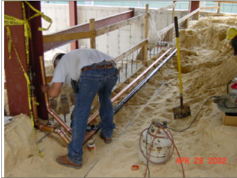
Gray water pressure lines
