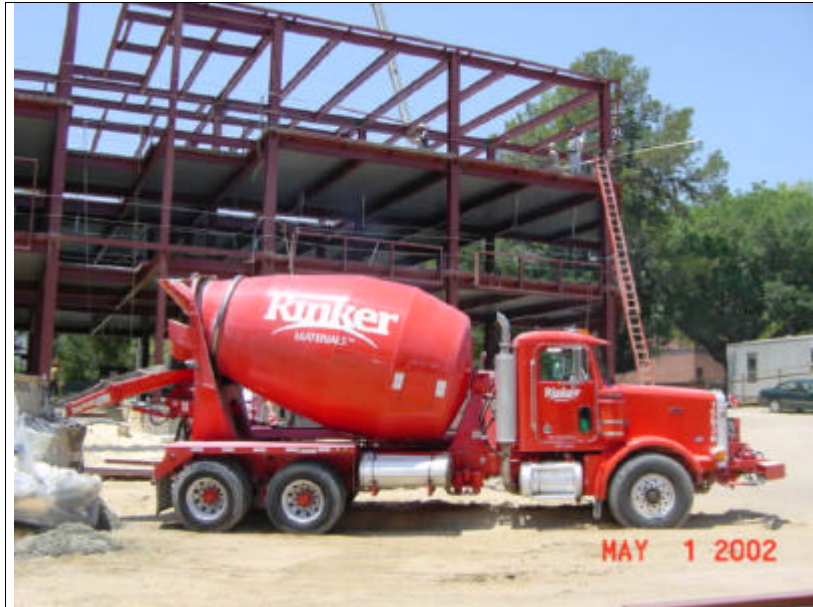
Rinker at Pump 2
