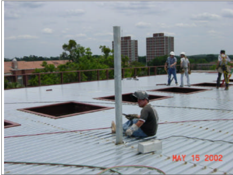
Lightning Preventer Mast
