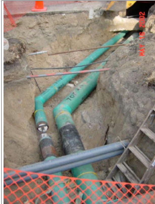
Steam lines at Manhole
