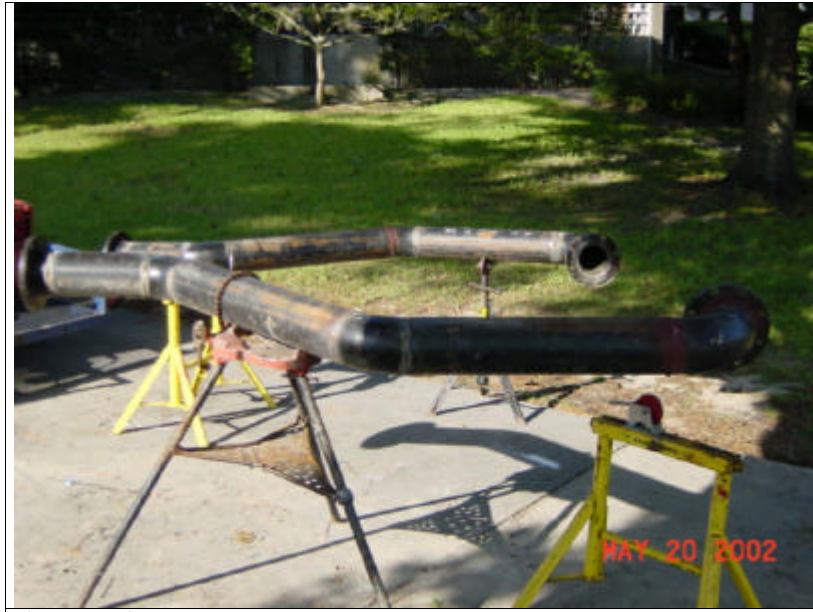
Pipe for Chilled water
